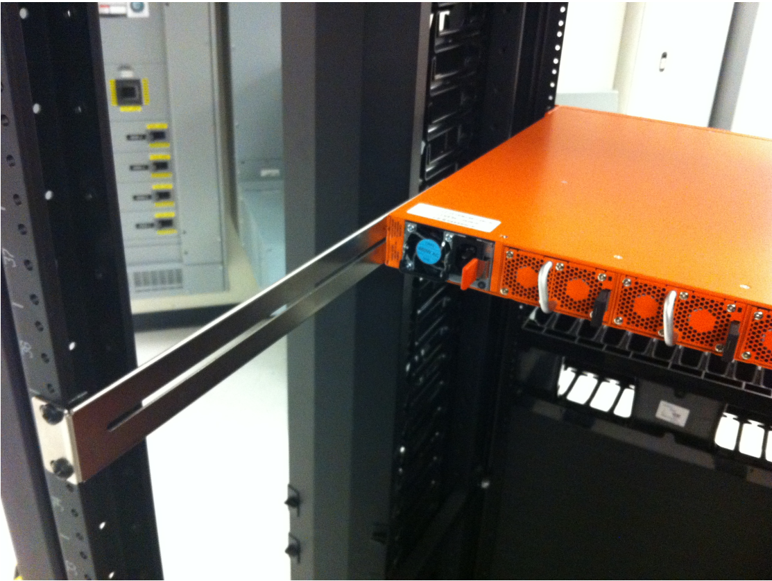
Figure 4 Rear View of the Mounted Node and Rails on the Four-Post Rack
